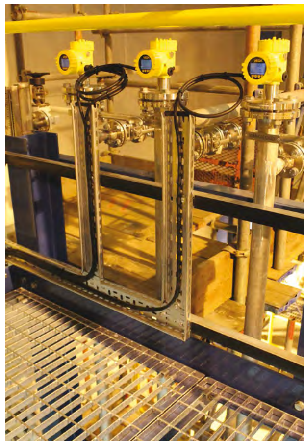
Direct measurement of the boiler condensate vessel level with VEGAFLEX GWR in bypass chambers.
