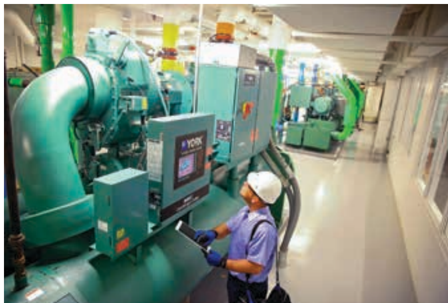
For owners of newer chillers, built-in features such as performance monitoring, an always-on connection to the IoT as well as self-identification of potential operating issues, offer big advantages.
