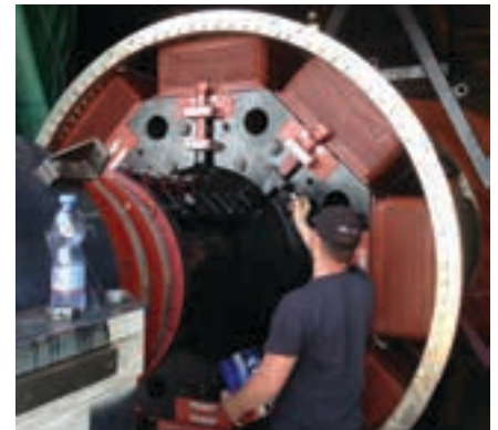
Marthinusen & Coutts Lead Field Services Technician, Wynand Willemsse applies finishing touches to one of the SNEL 70 MVA synchronous condensers completely refurbished in the DRC.
