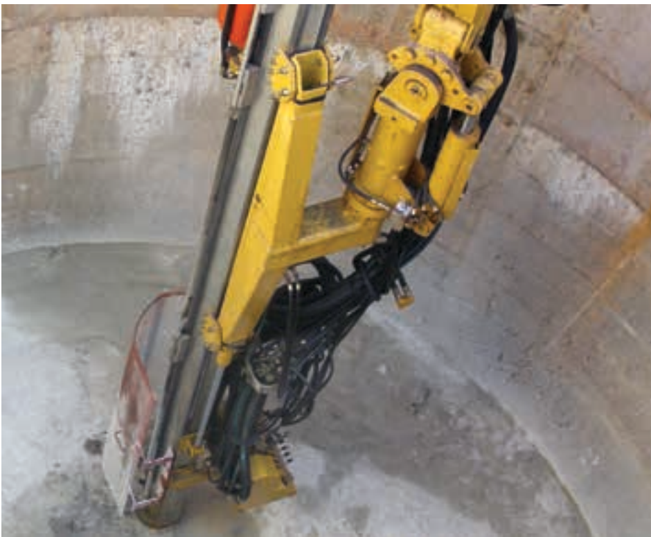
The shaft-sinking component at the Murray & Roberts Cementation Training Academy encompasses the pre-sink as well as the main sink.
