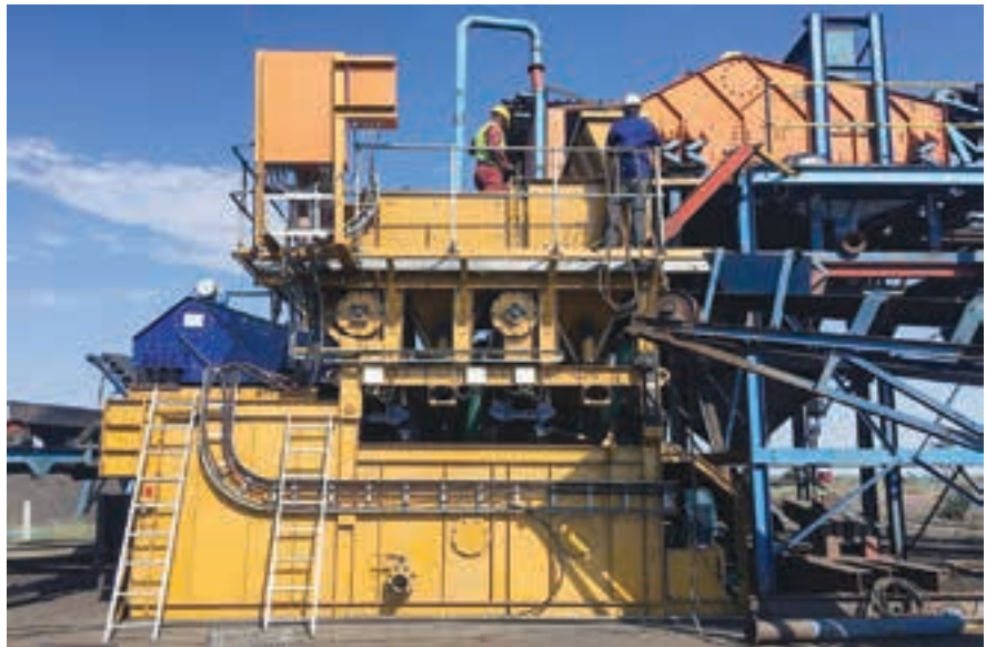
The new 100 t/h jig plant on site at the Otjo project (photo: Shaw River).
