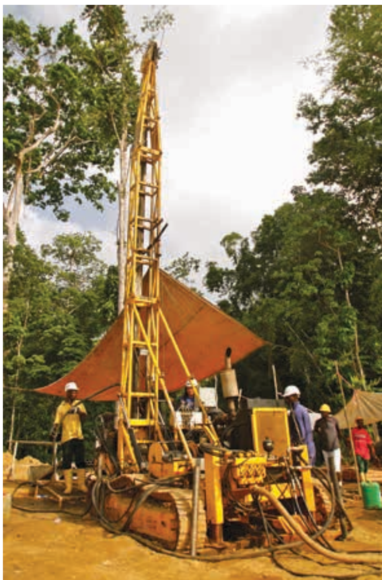
A core drill working at Dugbe. The project already has a 4,2 Moz gold resource and is said to have significant exploration upside.
