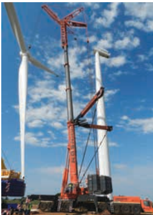
Some of the most technically challenging lifts being undertaken currently by Johnson Crane Hire are for the wind-energy industry, where loads of up to 100 t have to be lifted as high as 80 m.
