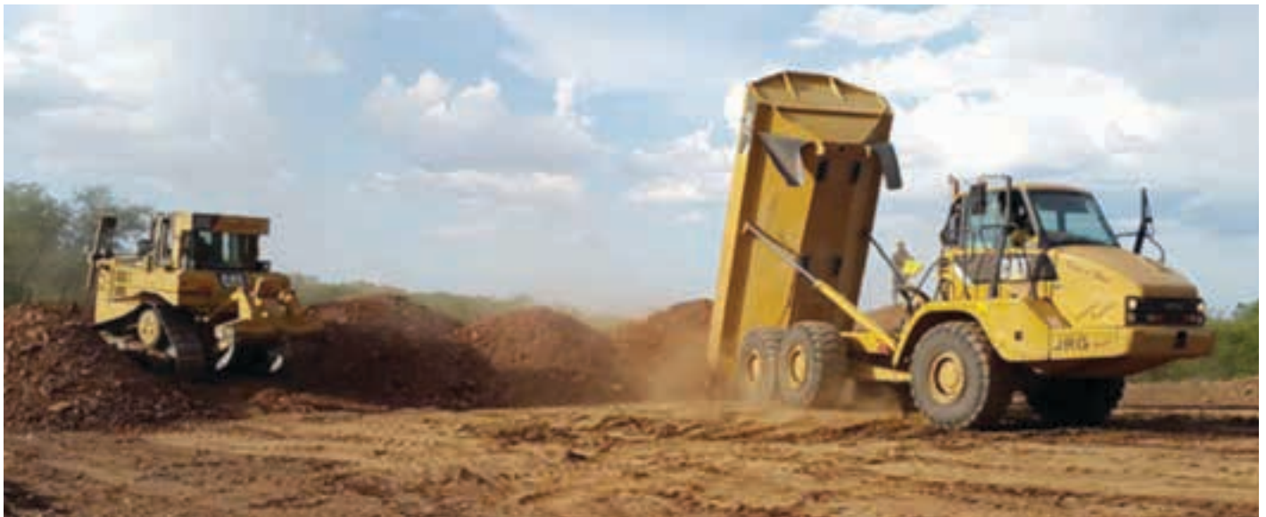
ROM pad construction at the RHA project nearing completion (photo: Premier African Minerals).
