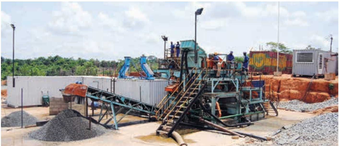
The 5 t/h bulk sampling plant at the Tongo Dyke-1 kimberlite project (photo: Stellar Diamonds).
