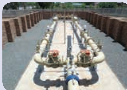
Recently certified to ISO 3834, AWS Pipelines offers qualified and professional services in the area of welding and pipe fitting to the petrochemical and manufacturing industries.
