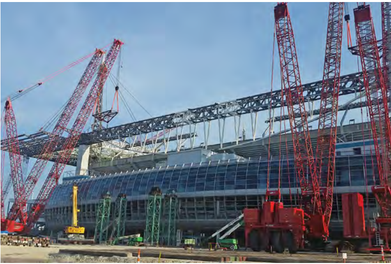
A fleet of Manitowoc cranes is helping a US contractor get the better of a challenging lift project.
