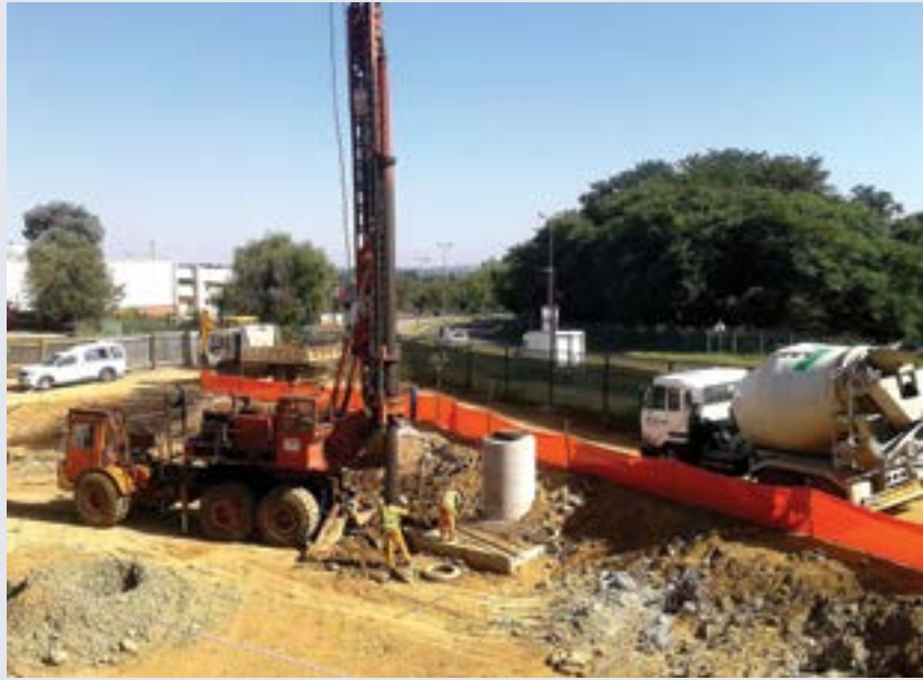
Gauteng Piling pictured in action providing the foundations for extensions to the Cresta Shopping Centre.
