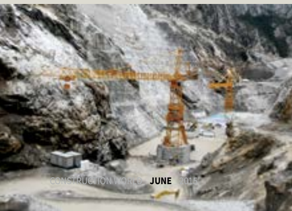
Potain tower cranes are used on large dam projects throughout the world.
