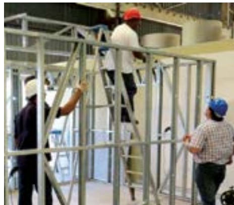
Willem Venter from Lafarge Gypsum explaining the correct installation of gypsum board.
