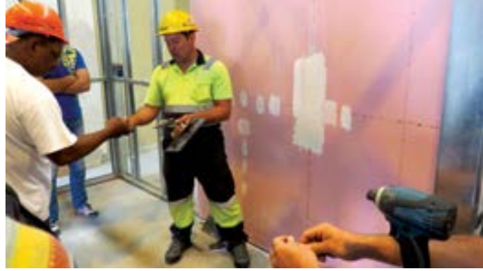
The 24 m 3 house that was erected by the students as part of the training course.
