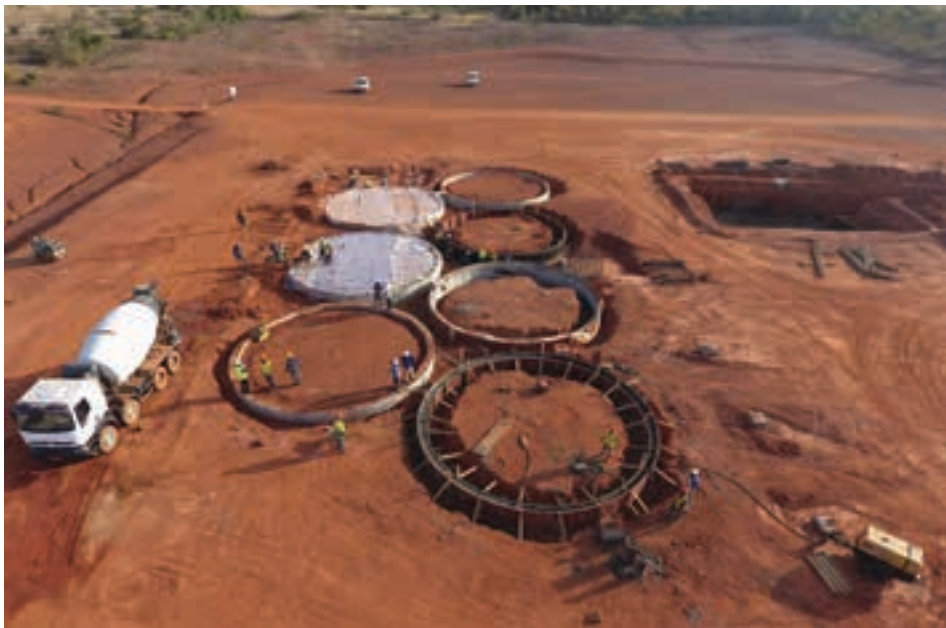
A recent view of the Yanfolila site showing the start of construction operations. The first concrete pour was in October (photo: Hummingbird).
