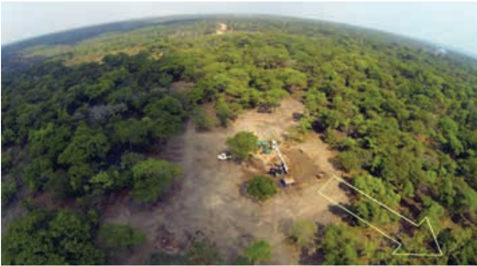
Geotechnical drilling at the planned Kakula boxcut location. Approximate direction of the planned access tunnels shown (photo: Ivanhoe).
