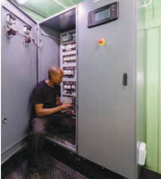
Chris Ngobeni, winding assistant at Marthinusen & Coutts, performing final checks on the generator rotor panel.
