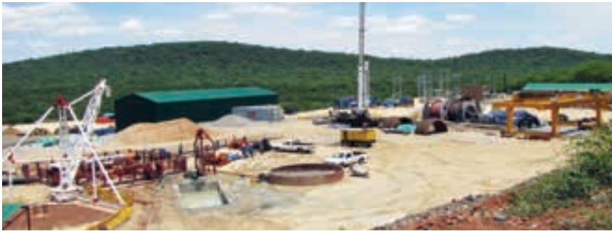
The central shaft site at Blanket as it was early last year. Shaft sinking reached a depth of 534 m by the end of 2016 (photo: Caledonia).
