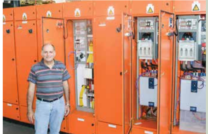
Santos Ferreira, Product Development Specialist at Shaw Controls, facilitated the testing of the Motor Control Centre (MCC) panels submitted for IEC testing.
