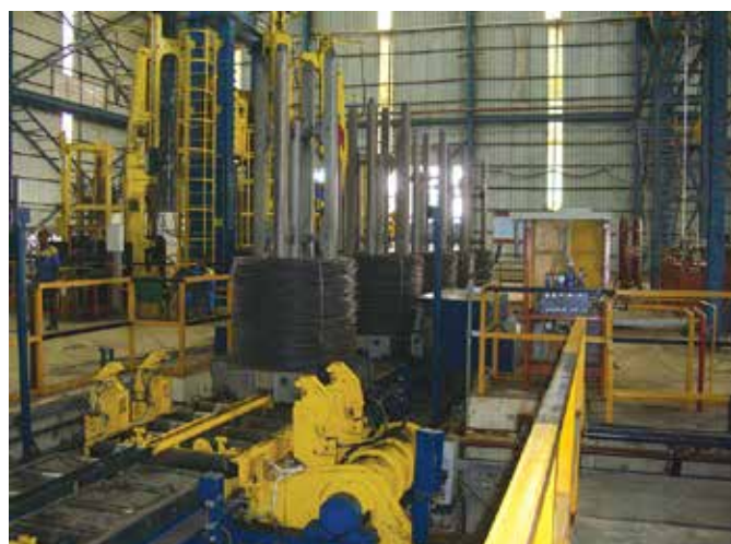
▲ Full production capacity is expected soon after Danieli completed its commissioning activities at Wempco's new wire rod mill
