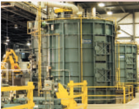
The basketless heat treatment system from Can-Eng Furnaces
