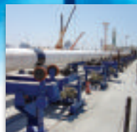
Spool base facility
