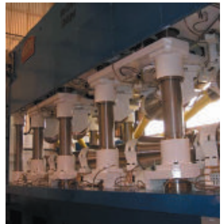
10 A 10-roll straightening installation from Bronx/Taylor-Wilson
