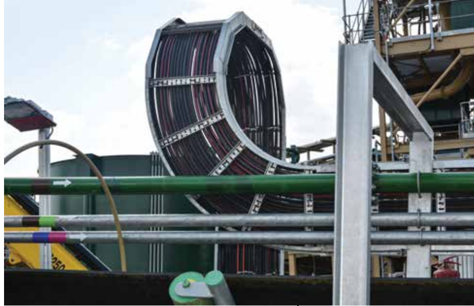
Creative cabling rack installation by Enl Electrical at Maseve Platinum.
