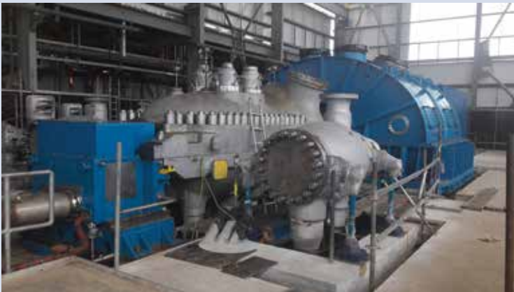
The turbine generator set showing the Siemens 150 MW generator and the low pressure and high pressure Skoda Doosan turbine set.
