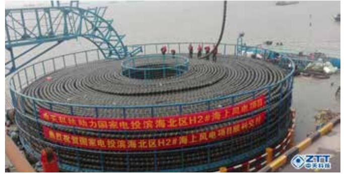
The 220kV submarine composite cable for the Binhai North Phase 2 offshore wind farm in Jiangsu province, China
