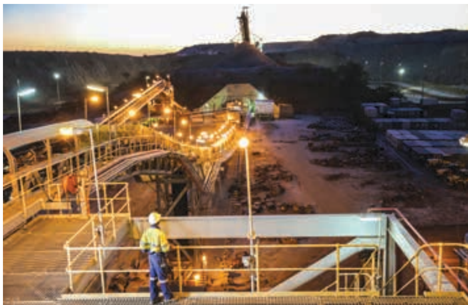
Acacia's Buzwagi mine is a low grade bulk deposit with a single large open pit. The process plant is designed with a throughput capacity of 12 000 tonnes of ore per day (photo: Acacia).
