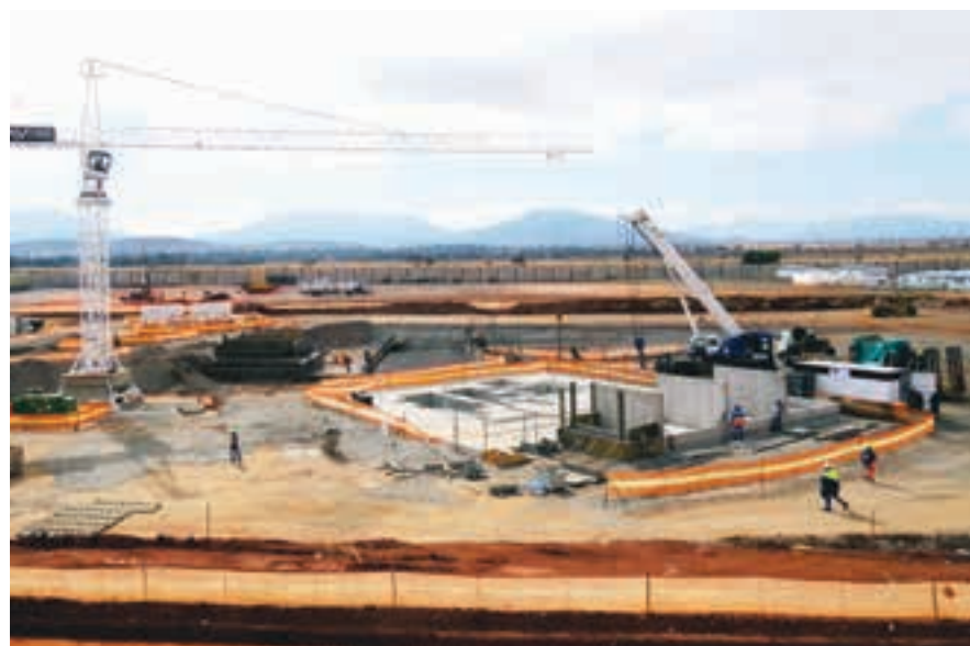
A recent view of the Platreef site, where the sinking of one of the shafts required for the project has already started.
