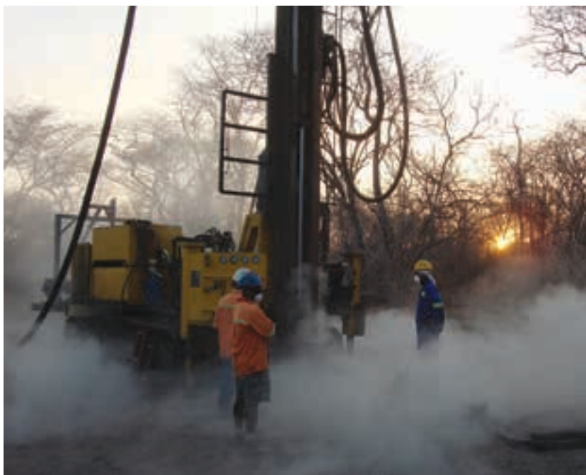
Drilling at the Mbeya Coal to Power Project site in Tanzania (photo: Kibo Mining).
