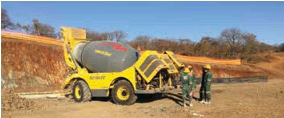
A concrete pour in progress at the Central Shaft site at Blanket (photo: Caledonia Mining).
