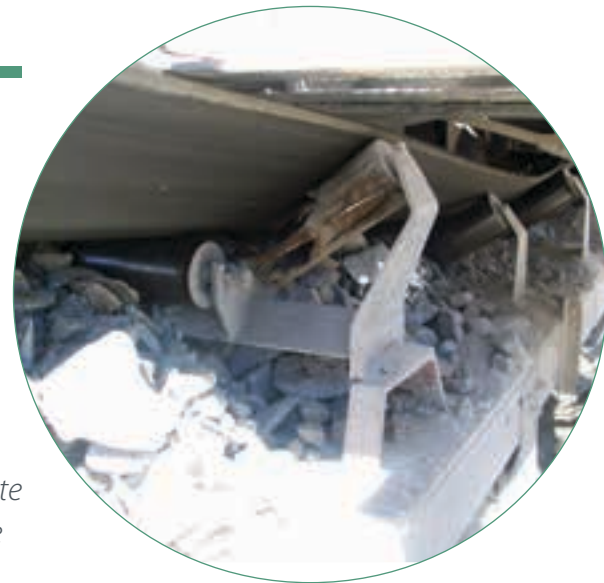
Are our conveyor systems still a workplace hazard? Looking at this photograph taken two years ago at a South African operation, they very definitely are (courtesy Marius van Deventer).
