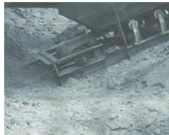
Figure 6: Unguarded pulley [4]. This is a completely unguarded tail/take-up pulley and loading area on a shot conveyor in a US quarry operation. In addition to the lack of guards, there is considerable material build-up below the conveyor. Any attempt to remove the material while the belt is running would require working in very close proximity to the nip point.
