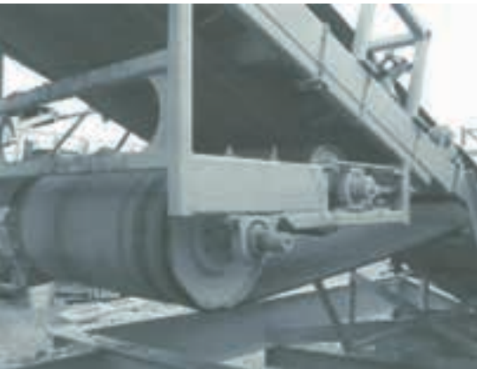
Figure 8: Another unguarded installation in a US operation that includes two unguarded pulleys. In this particular installation, it is clear that as well as no guards being installed, there are also no nip guards. There is in fact, no evidence of nip guards in any of the other referenced installations.
