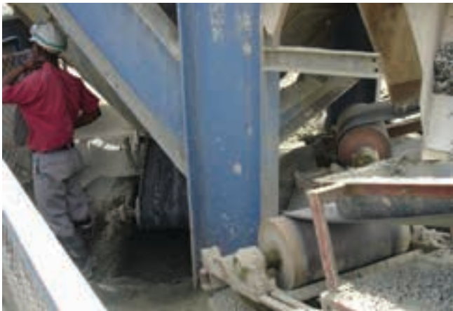
Safety incident in the making (courtesy Marius van Deventer).
