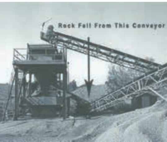
Figure 10: No safe crossing below the belt [4]. This is an installation in a sand and gravel operation, where a fatality occurred due to a large rock falling off the conveyor onto a person below the belt. Despite the steepness of the conveyor, it is clear that no effort has been made to prevent access to the danger area underneath, or to provide a safe underpass, where required.
