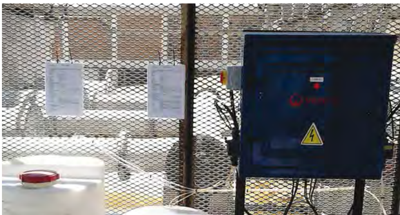
Veolia installed spill-proof and accurate chemical dosing stations around the mine.
