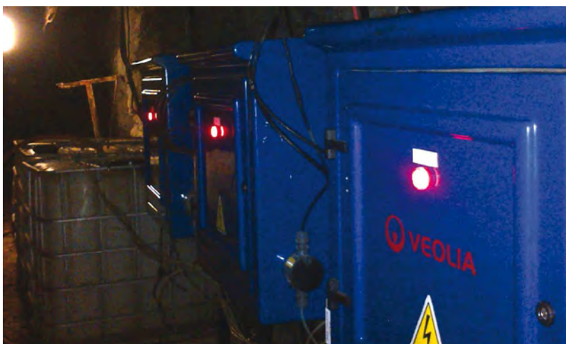
Veolia designed and installed 12 new treatment stations situated above ground and 1,8 km below ground that increased the mine's overall efficiency.
