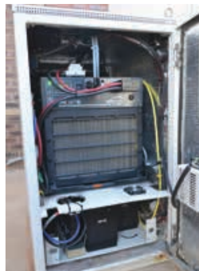
A 5.0 kW Altery FPS Fuel Cell supplied by Powertech Systems Integrators (PTSI) has been installed at Windsor East Clinic in inner Johannesburg, along with a hydrogen supply and monitoring service from Air Products South Africa.
