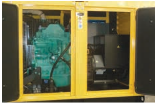
Zest WEG Group's Generator Set Division is able to offer solutions from a single diesel driven generator (seen here) to total standby power solutions.
