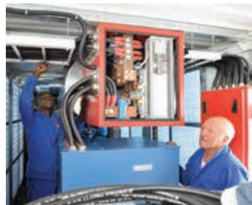
A view inside a containerised generator set from Zest WEG Group's Generator Set Division.
