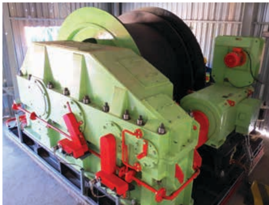
Shaft 1 winder ready for commissioning (photo: Ivanhoe).
