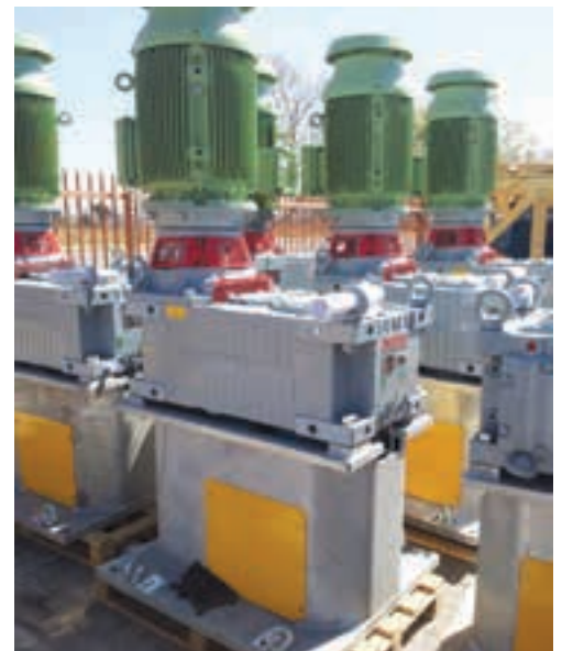
The acid mine drainage plant consists of a combination of 53 specialised Mixtec mixers.
