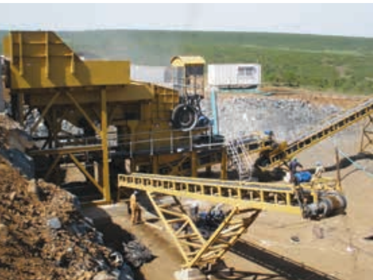
The extensive range of Trio equipment allows Weir Minerals Africa to offer customer crushing solutions.
