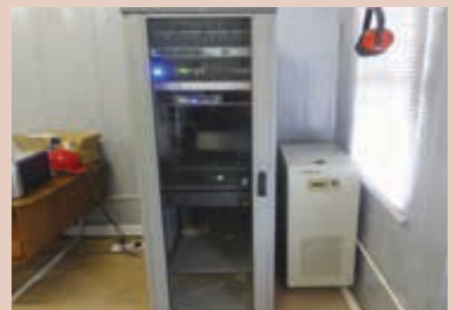
Satellite receiver, network switches and VoIP PABX installed in the Lerala office are the ‘brains’ of the new communications system.
