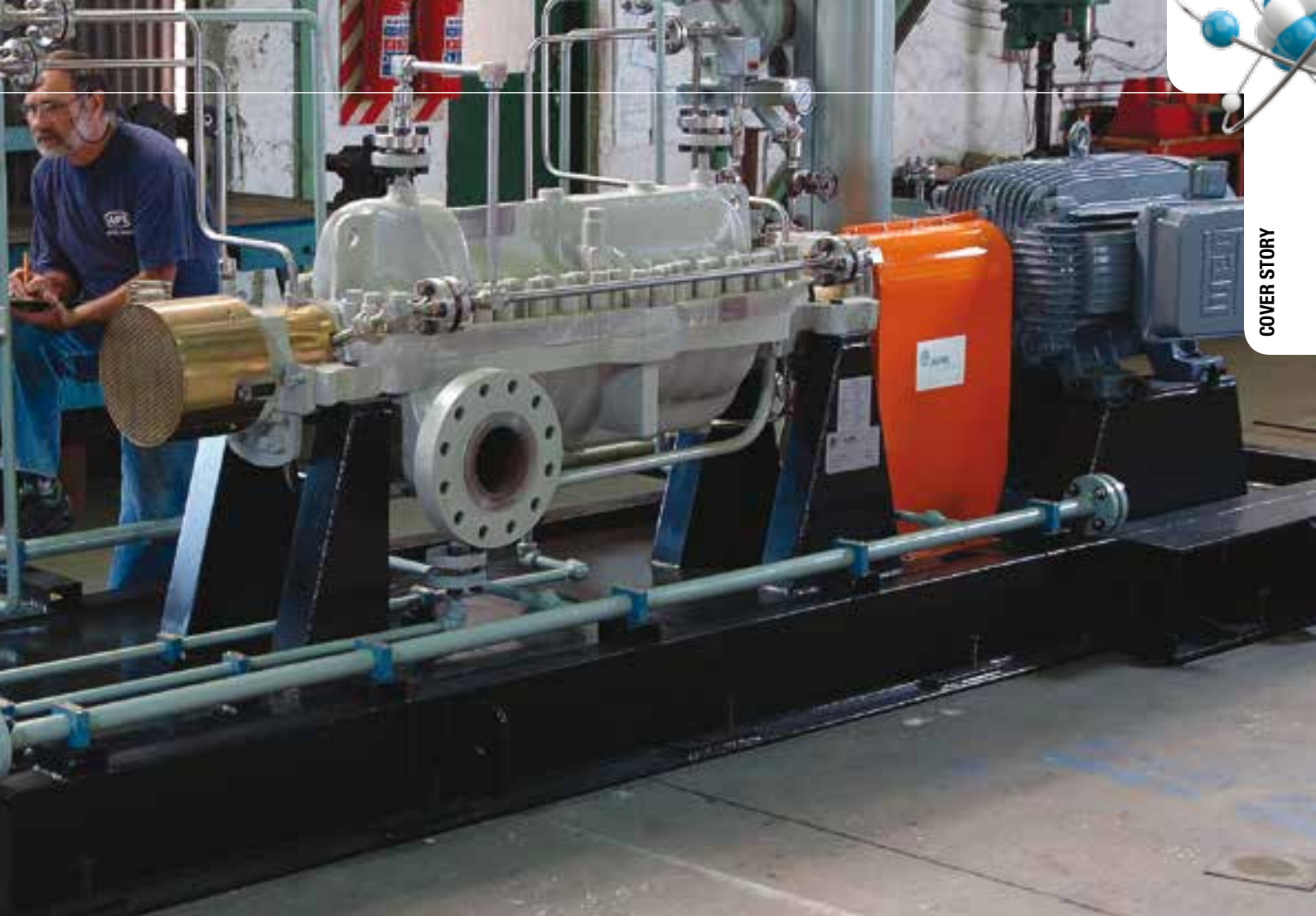
An API 610 multistage petrochemical pump installed in Harrismith for Petro SA.
