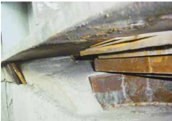
Figure 3: Grouting and support blocks in this example are very poor.
