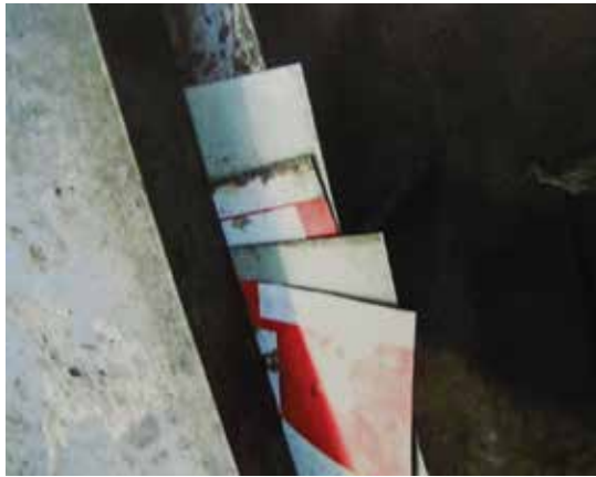
Figure 6: Example of poor shimming using scrap metal.
