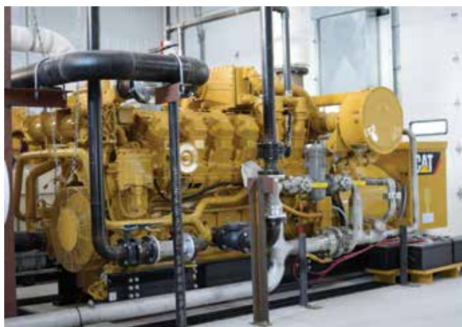
An example of a project undertaken internationally by a Cat dealer involving two G3512 biogas generator sets to produce electricity.
