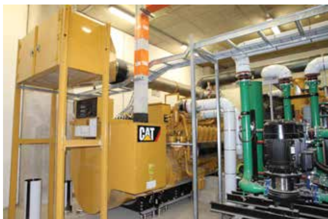
The gas engine power plant supplies one fifth of the electric power for the new Standard Bank building, with generator set's thermal energy recovered for the bank's hot water and air conditioning requirements.
