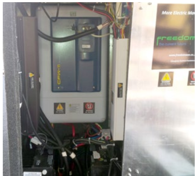
Figure 4: 88A CFW 11 mounted into the Chobe Game Lodge electric boat (Freedom 4) console along with the battery management system, chargers, 12 V battery and other electrical equipment.
