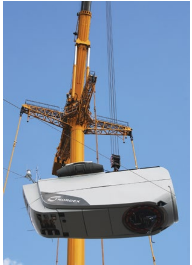
Figure 1: Nacelle housing gearbox and generator being hoisted during installations (courtesy of Nordex).
