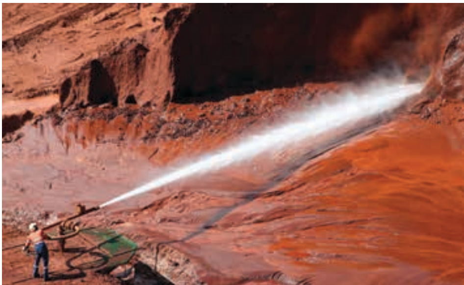
The hydraulic mining unit (HMU) in operation at Kwale Central Dune (photo: Base Resources).
