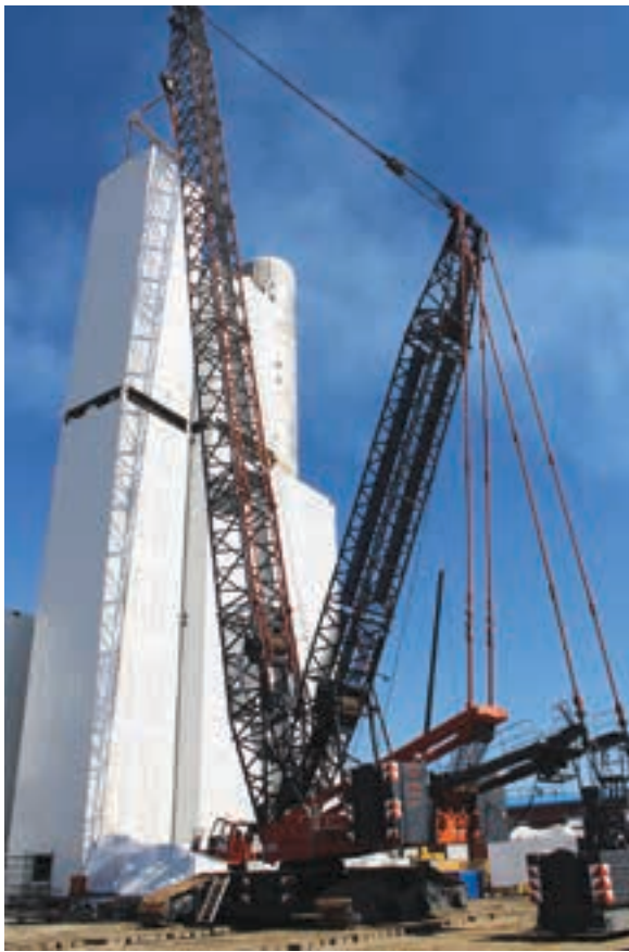
Most of the large components were lifted in an almost fully assembled state.
