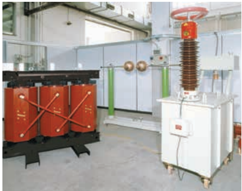
Cast-resin transformers in the test bay.
