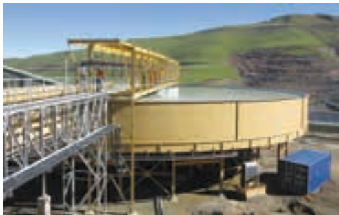
A typical MIP installation. The company is currently manufacturing linear screens and a clarifier for an Australian customer in Panama at its factory in Springs.
