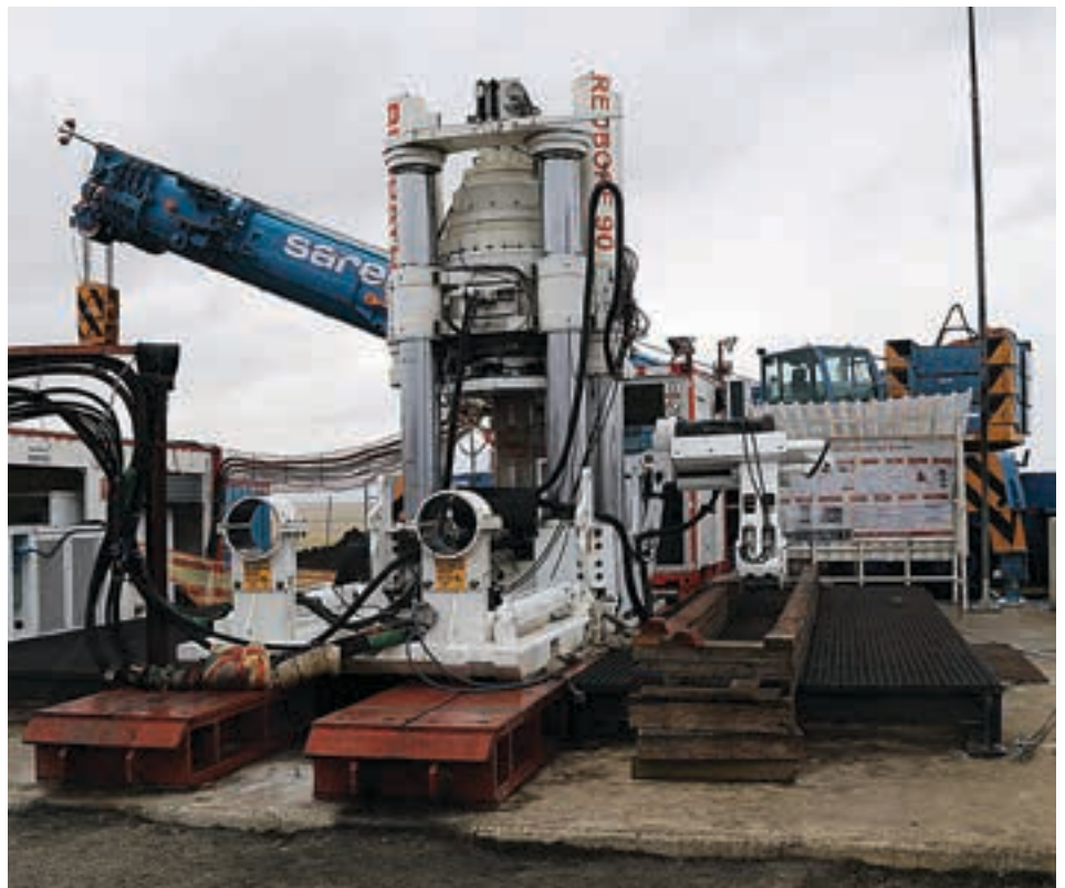
The Redbore 90EX deployed by Redpath at Sasol's Impumelelo mine (photo Redpath Mining).
