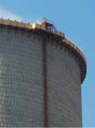
A view of the completed access platforms running around the circumference of the 165-metres high cooling tower.
