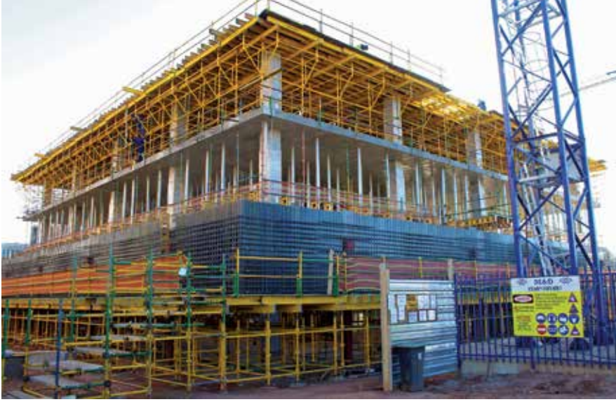
The off-shutter external and internal finish inside the structure will make it the central focus on the university campus.
