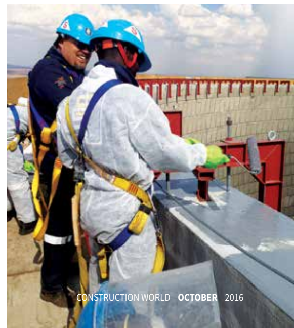
Polyurethane coating is applied to the top rim of the cooling tower.
