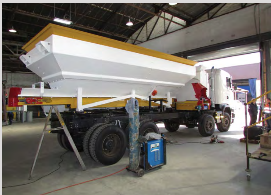
A stemming truck under construction at Cobra Petro Project's facility in Johannesburg.
