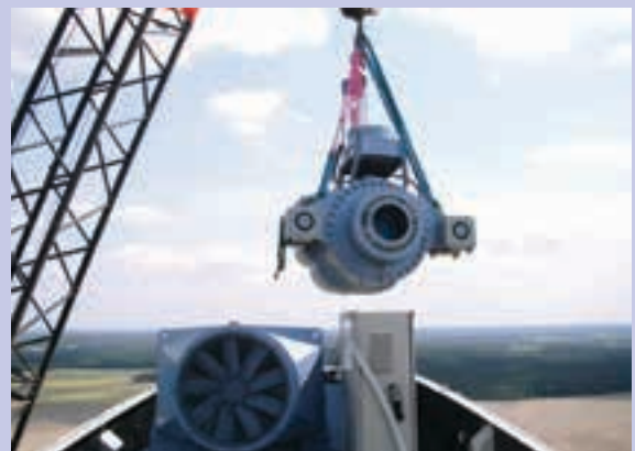
A service team from seebaWIND exchanges the gearbox of a wind power plant in Poland.
