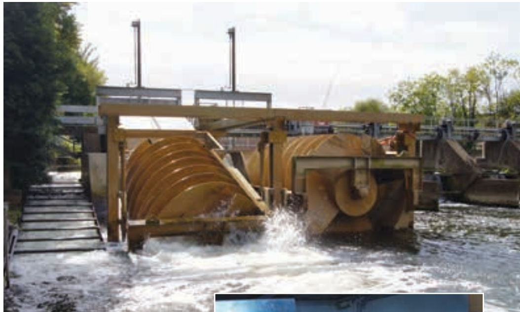
Above: A mini power station installed on the River Thames at Romney Weir produces 'green' electricity by means of water-driven Archimedes screw generators based on two WEG W22 premium efficiency IE3 generators.
