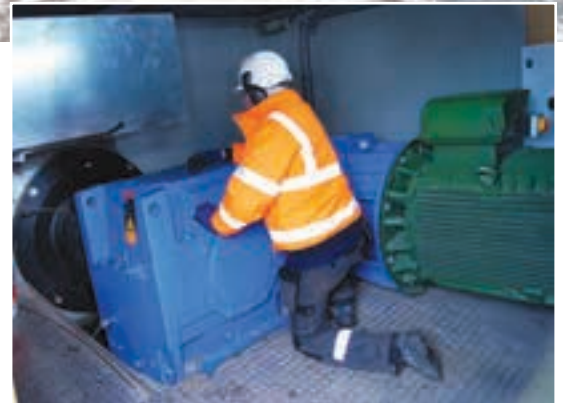
Right: The W22 units are 'special' products for this application in the sense that they are generators based on a W22 motor. At 96% efficiency, they were a critical part of the power transmission design to ensure the six-year return on investment target was met.
