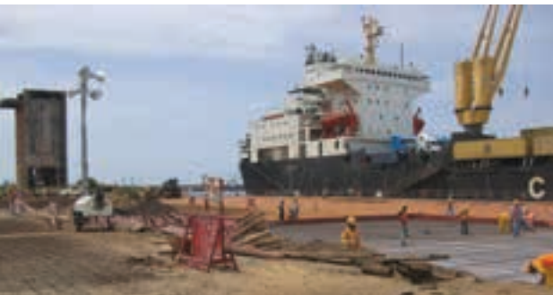
The Zest WEG Group's Enl Electrical will construct 6.6 kV overhead power lines for a ship loading facility at the Port of Buchanan in Liberia.
