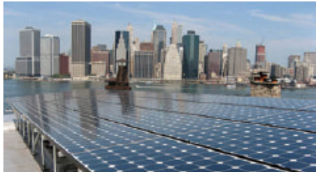
○ Solar Energy Systems installed this solar PV rooftop system in New York City. Photograph courtesy of Aeon
