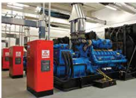
Six 2 000 kVA open type synchronising generator sets
