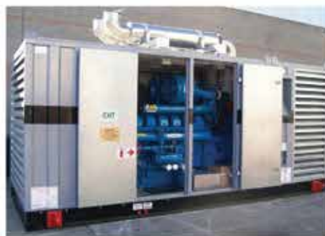
Containerised 1 250 kVA generator set
