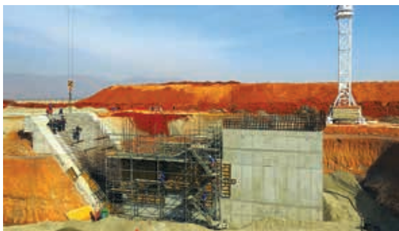
Collar construction in progress for the 975 m deep, 7,25 m dia Shaft 1 (photo: Ivanhoe).
