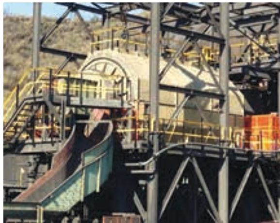
A typical Osborn rotary breaker installation.
