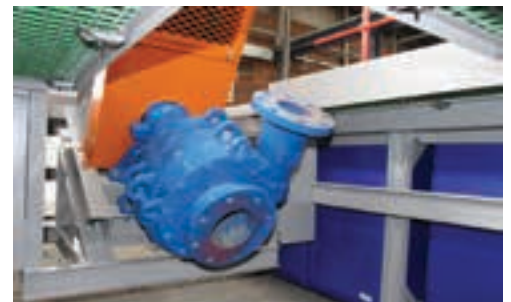
One of two Warman DWU 125 dewatering pumps mounted to a pontoon and walkway during assembly phase.
