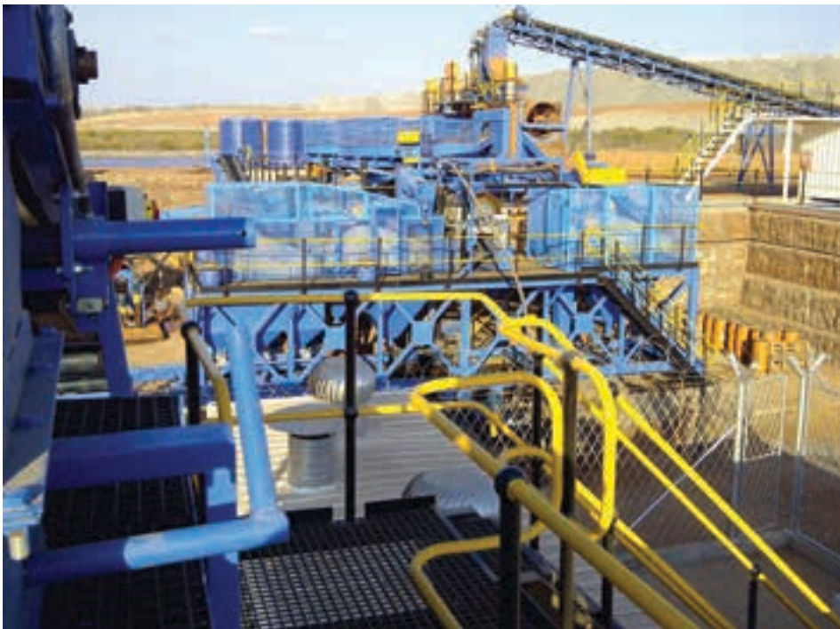
The main processing plant at the Krone-Endora at Venetia project (photo: Diamcor).
