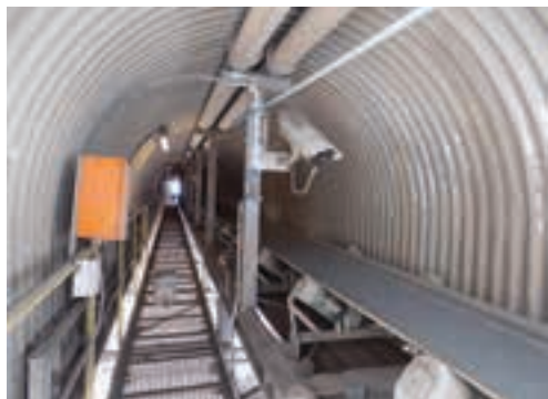
Land Arc thermal imaging cameras installed at a lime manufacturing plant in the Northern Cape.
