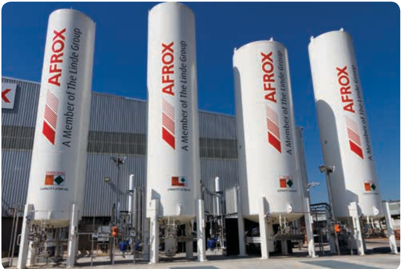
Four cryogenic storage tanks dominate the Riverhorse Valley skyline. The plant takes delivery of liquid CO 2 , Nitrogen, Oxygen as well as Argon from Pretoria.
