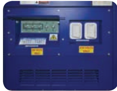
In addition to the welding units, 30 kVA three-phase power and two 6.0 kVA, 230 V power outlets are accessible for supporting activities such as heat treatment and grinding.
