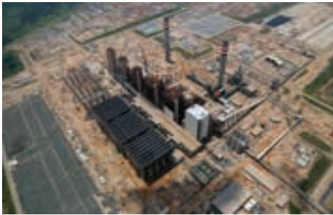
Babcock's has secured a contract extension for Units 4 and 5 for the balanced erection of high-pressure pipework systems for the 800 MW boiler units at Kusile Power Station.
