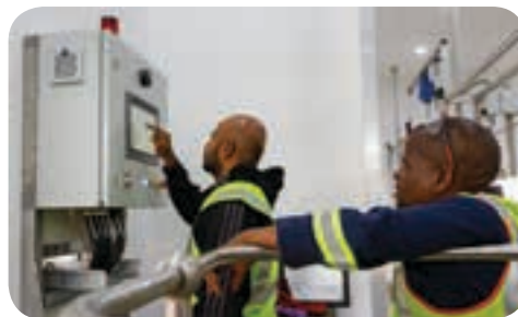
The operator attaches a manifold of cylinders to the filling station, selects the recipe required from the SCADA and the PLC will automatically fill the cylinders to the correct composition.
