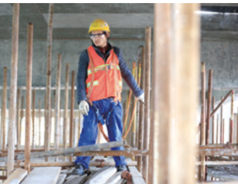
A new unit to manufacture label materials and speciality papers is under construction at the Changshu mill in China.
