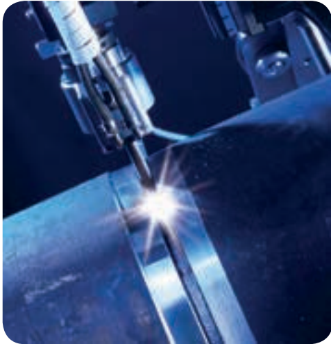
Narrow gap hot wire TIG welding is emerging as an essential technique for joining critical components such as those required for the ITER, mooted to be the world's largest tokamak fusion reactor.
