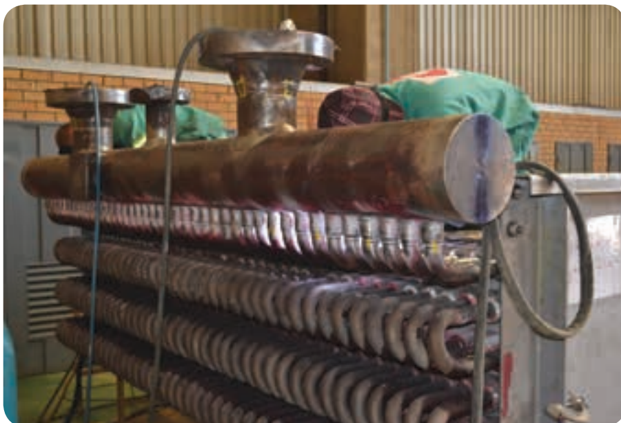
A heat exchanger for Natref under construction. The welders had to weld 585 U-bend joints per bundle, nearly 1 200 tube-to-tube butt welds, and achieved a very low weld repair rate – an impressive feat when mirror welding has to be employed.
