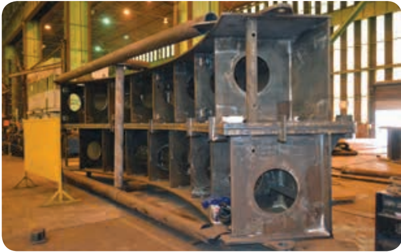
Dragline bases are complicated structures that require significant numbers of internal stiffeners. After completing the assembly, the accuracy required has to be “within 6.0 mm across the 17.7 m diameter, in terms of flatness and roundness.”
