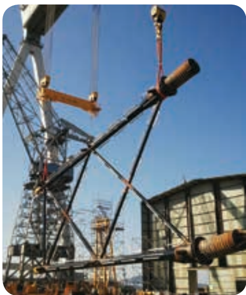
Undertaken by a Spanish company, seamless flux-cored wire from voestalpine Böhler Welding was used in the construction of the support structures.
