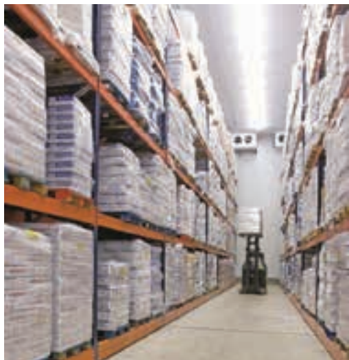
APC Storage Solutions SA has designed a cold storage facility for Lynca Meats, consisting of a Movirack® mobile racking system and two articulated forklifts.
