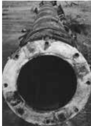
Figure 2: Bending of the column was clearly visible.
