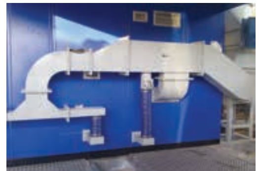
JB Switchgear approached RTS to supply dedicated back channel cooling to the VSD panels on the mine.
