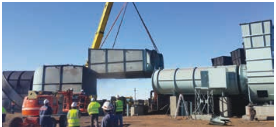
The retrofit involved having to remove the existing shaft top, replace it with a new one and make the entire system ready to go back into service on the morning of the fourth day.
