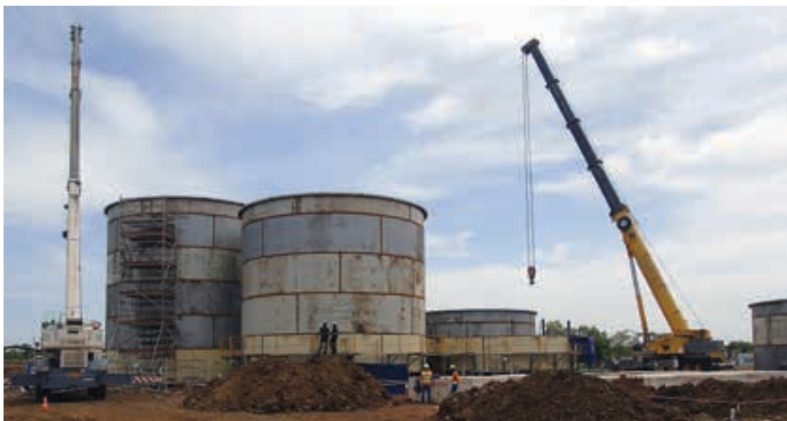
A recent view of leach tanks under construction at the Bougou site.
