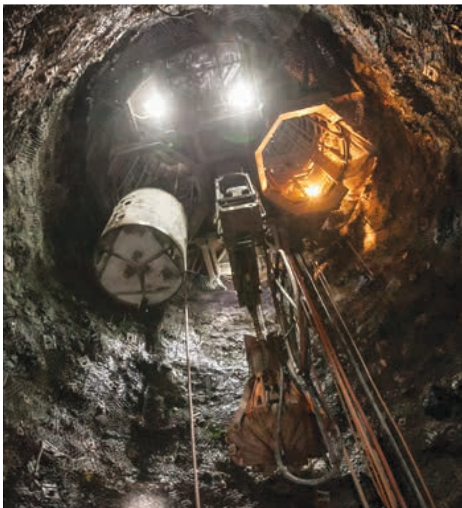
Inside Shaft 1. Sinking has now reached a depth of over 450 m below surface and is advancing at a rate of 45 to 50 metres per month.
