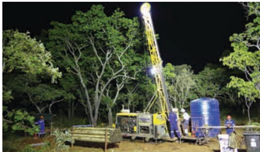
An Atlas Copco CS14 core drilling rig at work at Arcadia (photo: Prospect Resources).
