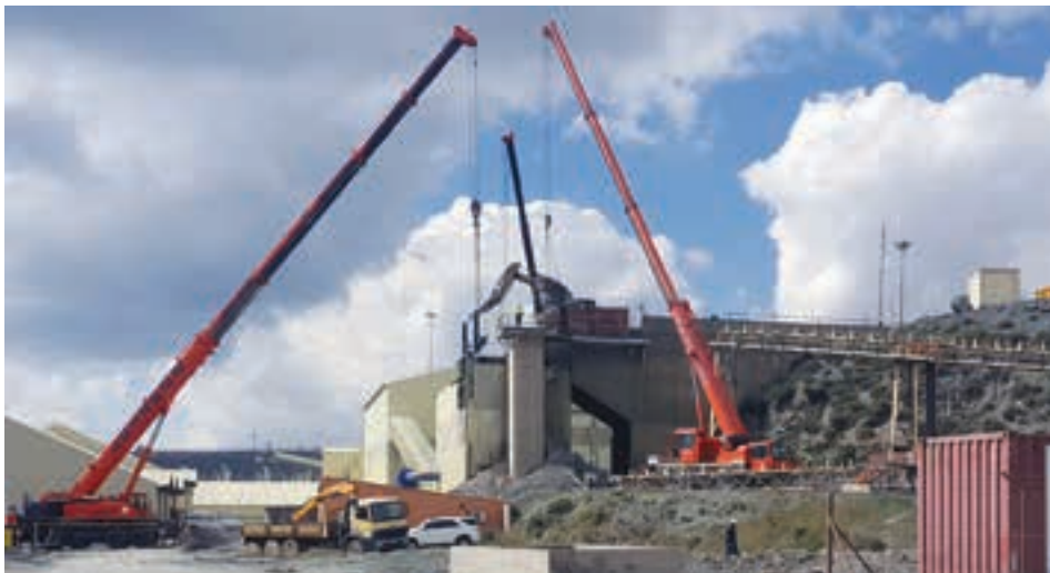
Johnson Crane Hire undertaking a lift on a mine site in Lesotho.
