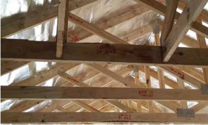
Truss hangers not installed due to a mix-up with a different section and detail.
