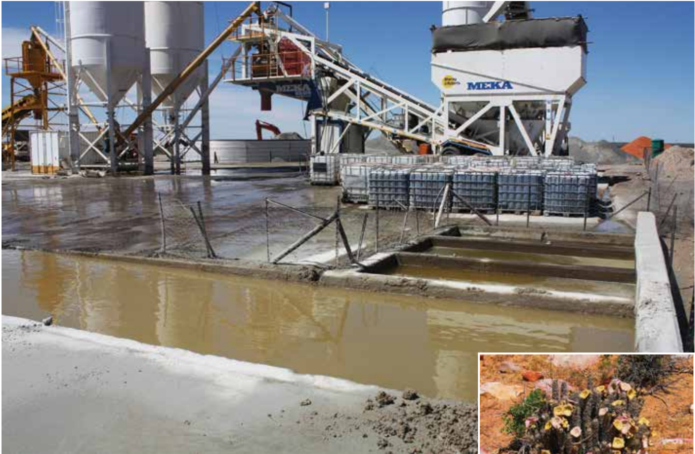
Another initiative aimed specifically at reducing water consumption was the construction of a specialised wash bay solution at the on-site batch plant.
