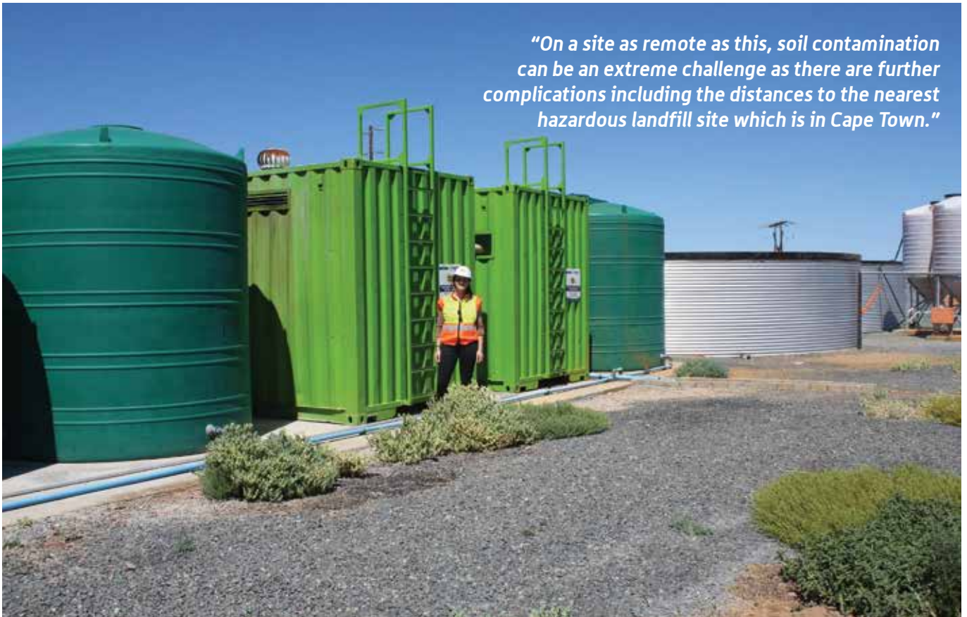
Marli van Rooy, environmental officer for Murray & Roberts Infrastructure, outside the modular water treatment plant installed by the company.
