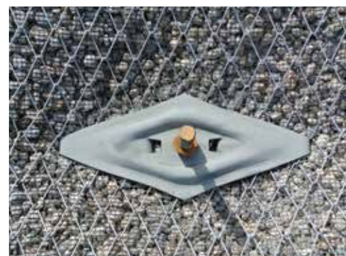
MAIN: Franschhoek Pass midway through the project. INSET: High-tensile steel wire mesh with newly developed large spike plate.
