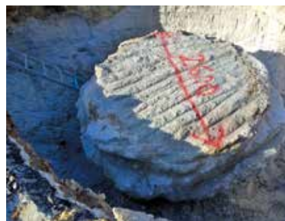
TOP TO BOTTOM: Installation of the sleeves to protect services from damage. Layout of jet grouting columns. Exposed trial column with a diameter of 2 600 mm.
