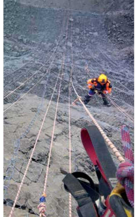
The project depended heavily on rope access technicians operating the Decoiler, as well as stitching close the drape wire mesh panels.
