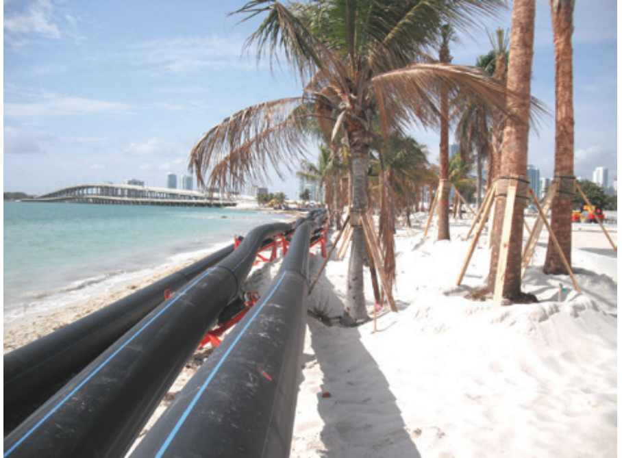
For a new water main in Miami, USA, 1,600 feet of 30" diameter PE 4710 HDPE pipe was installed 100 feet deep using horizontal directional drilling (HDD)
