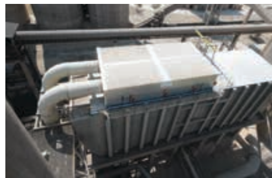
A bird's eye view of the reverse-pulse ESP conversion developed and installed by John Thompson Air Pollution Control at PPC's Dwaalboom cement factory near Thabazimbi.
