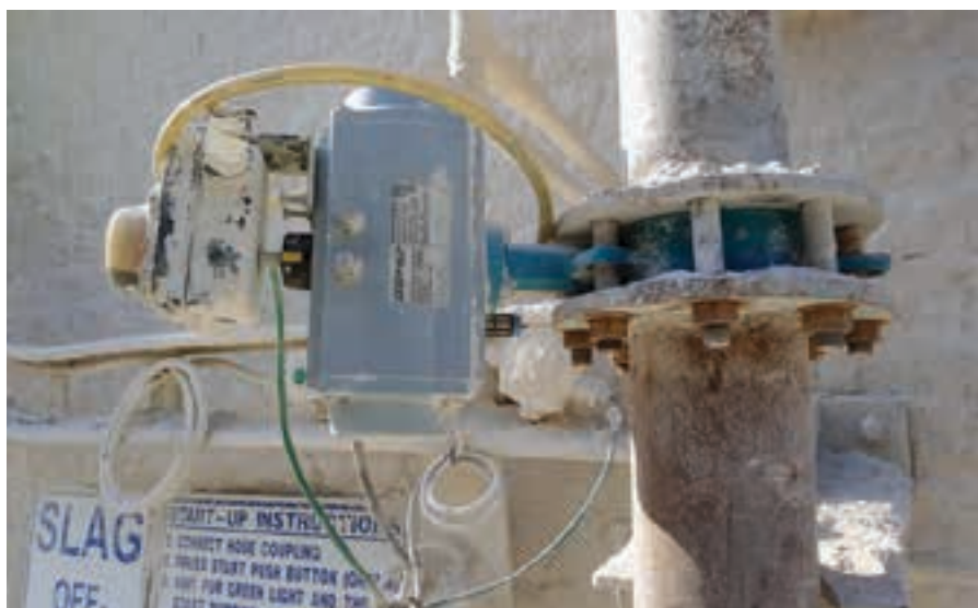
Gemü Valves Africa's four-inch soft-seated butterfly valve at one of AfriSam's cement blending and packaging plants.
