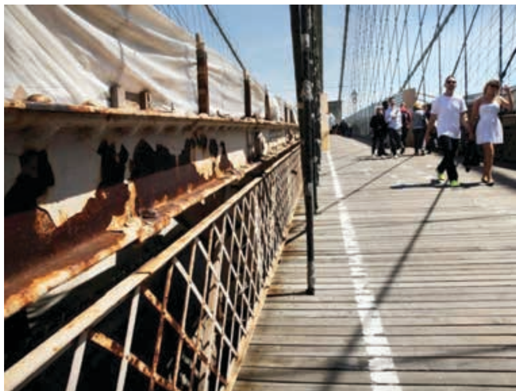
The repair of the Brooklyn Bridge in Manhattan, originally scheduled for completion in 2005, took until 2016 to complete and total costs of fixes and improvements rose more than US$600-million.
