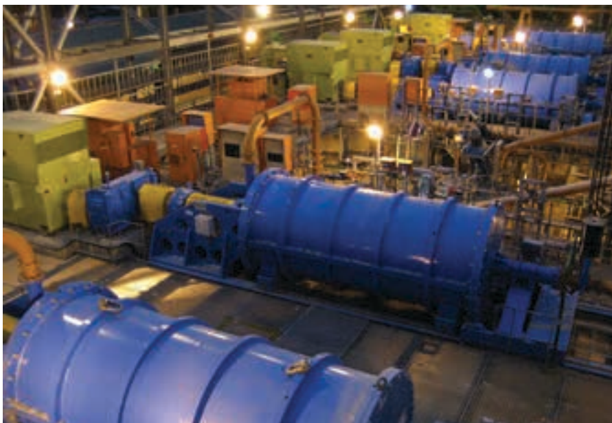
Glencore Technology's highly energy efficient IsaMills™ are now meeting the grinding requirements at Anglo Platinum's Waterval Retrofit plant.
