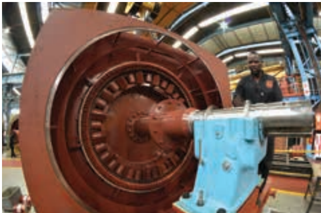
Alpheus Mtshali, from Marthinusen & Coutts, is pictured with the 1 586 kW 187.5 rpm, 3.3 kV, 278 A stator.
