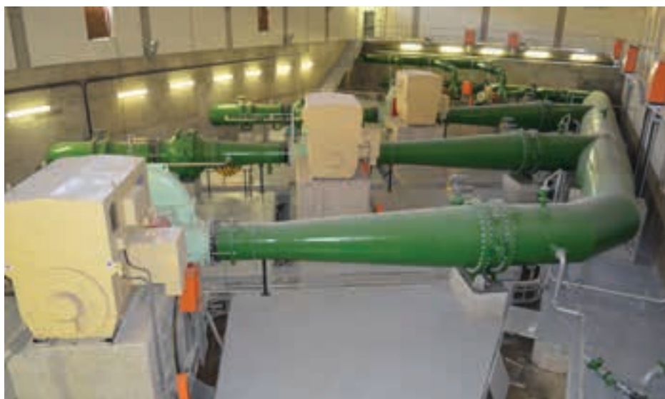
AECOM was responsible for the design monitoring the construction of the water transfer system that forms part of the Trans-Caledon Tunnel Authority's Mooi-Mgeni Transfer Scheme, which includes a 58 MW pump station to take water from Spring Grove Dam.
