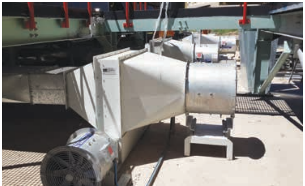
Back-channel cooling, along with RTS Africa's spin-filter technology, offer a cost-effective way of ensuring that temperatures within VSDs in motor control centres remain at safe levels.
