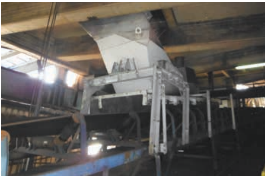
Operating with Weba Chute Systems in the Isdemir plant has seen the noise level decrease by more than 10 dB to 83 dB, which allows a period of eight hours at this level of exposure.
