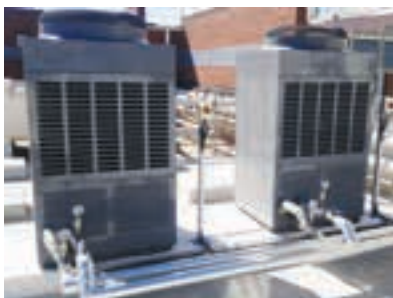
Two 40 kW industrial heat pumps installed by Magnet Energy.
