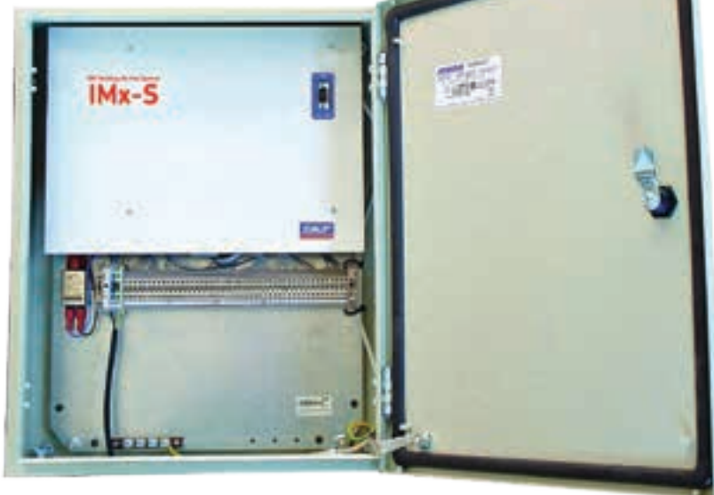
Below: A new coal mine in Limpopo has installed 78 condition monitoring systems based around the SKF IMx multi-log online condition monitoring unit.
