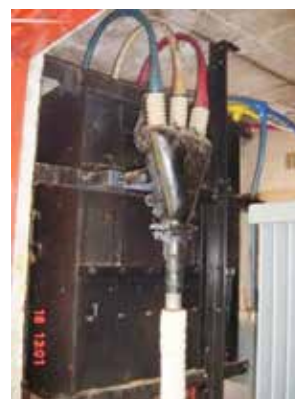
Figure 7: Compound filled cable boxes.
