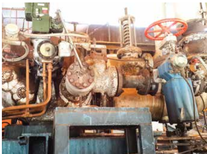
Figure 3: Mill steam turbine.
