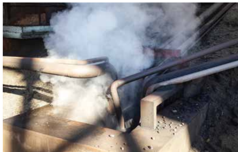
Figure 2: Steam drain pipes from the steam turbines.
