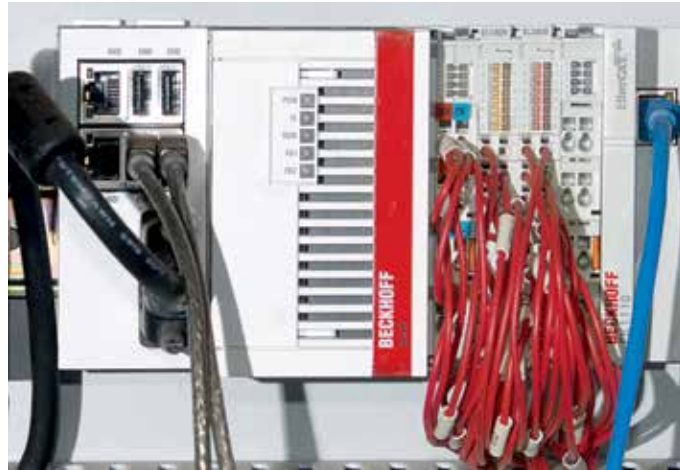
View inside the control cabinet of the CNC-800A3 with the CX5120 Embedded PC as the central control platform.
