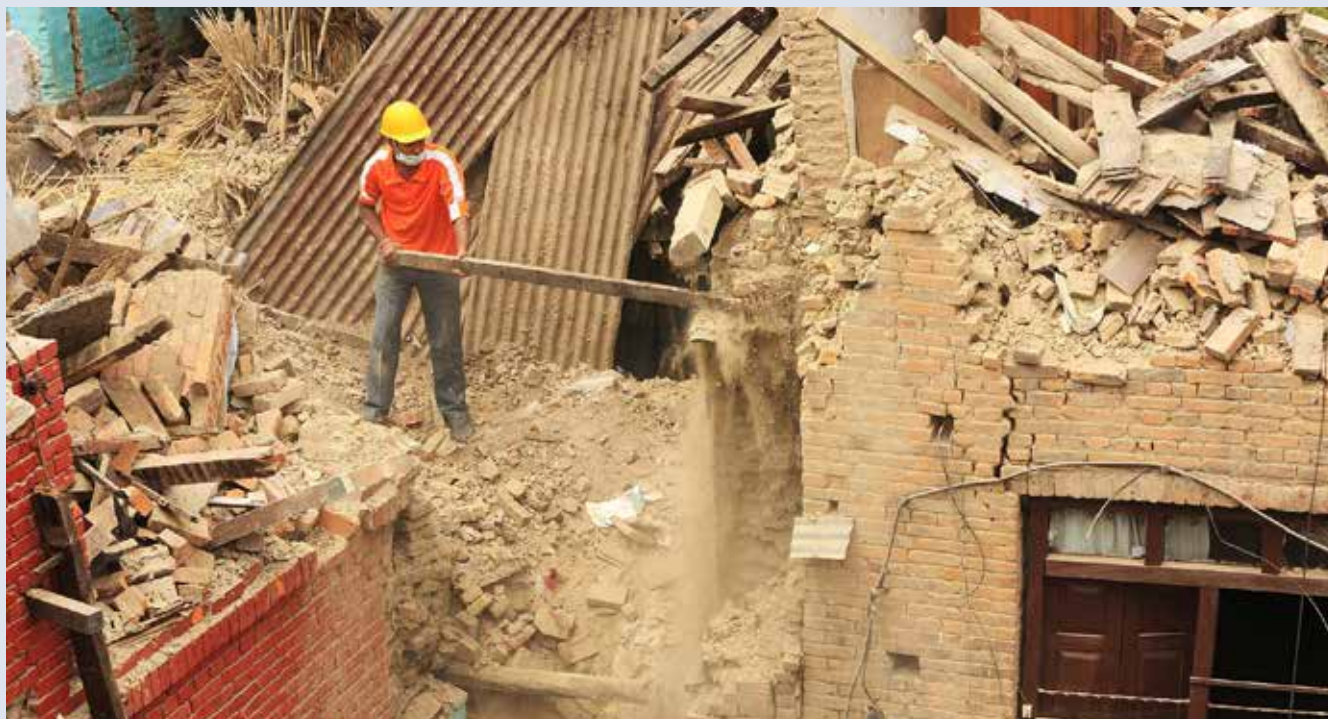
Earthquake damage in Bhaktapur. Photo © UNDP Nepal/Laxmi Prasad Ngakhusi
