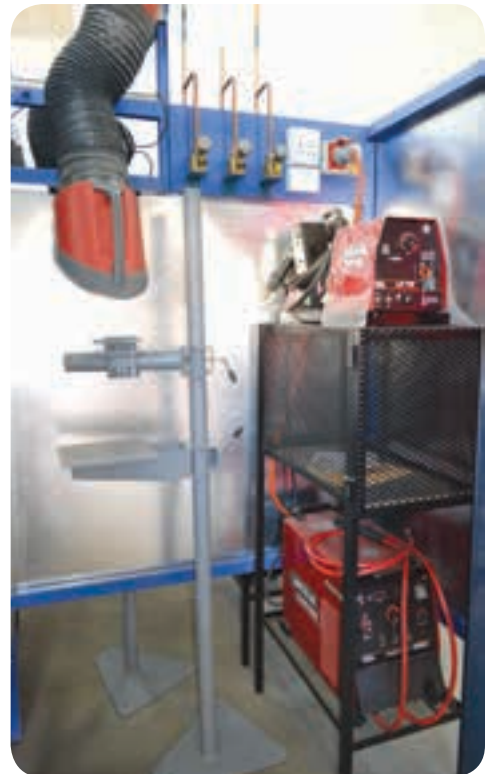
The welding bays at the Cosmo Training Academy supply three welding gas mixes via the Air Products CryoEase system: pure argon for TIG and aluminium GTAW welding; argon, CO 2 and oxygen mixes for GMAW welding of steel; and pure CO 2 for short-arc FCAW welding of steel.
