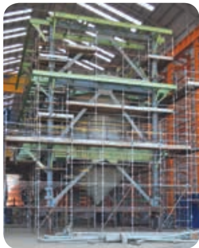
One of the 24 CTFE modules has a mass of over 400 t and includes two pressure vessels and all of the interconnecting piping, flanges and support structures.
