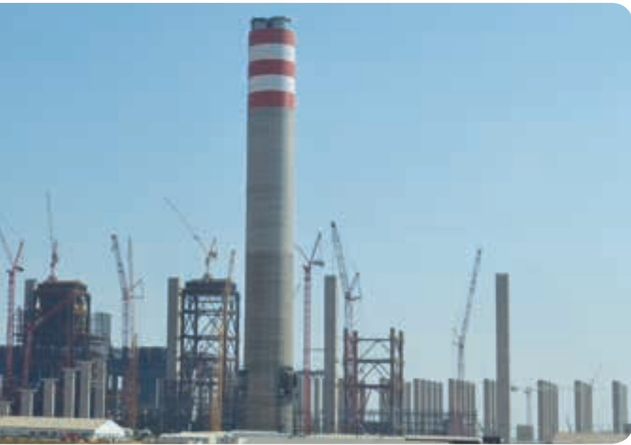
The Kusile power station under construction during July 2015. The erection of Unit 1 (left) is nearing completion and local component and structural steel fabrication is now complete, leaving South African fabricators facing difficult times.
