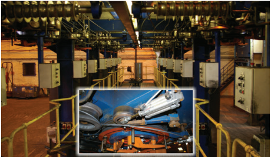
▲ Thorite-supplied control boxes in Bridon's Wire Mill & Ropery
