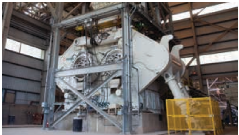
Another view of the HRC™ 3000, which has a total installed power of 11 400 kW and a total installed weight of 900 tons.
