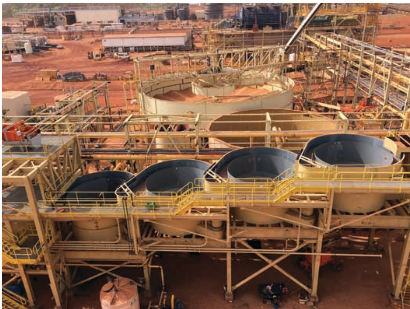
The Fekola plant under construction showing the leach thickener and the CIP section. The plant will have a throughput capacity of 5 Mt/a (photo: B2Gold).
