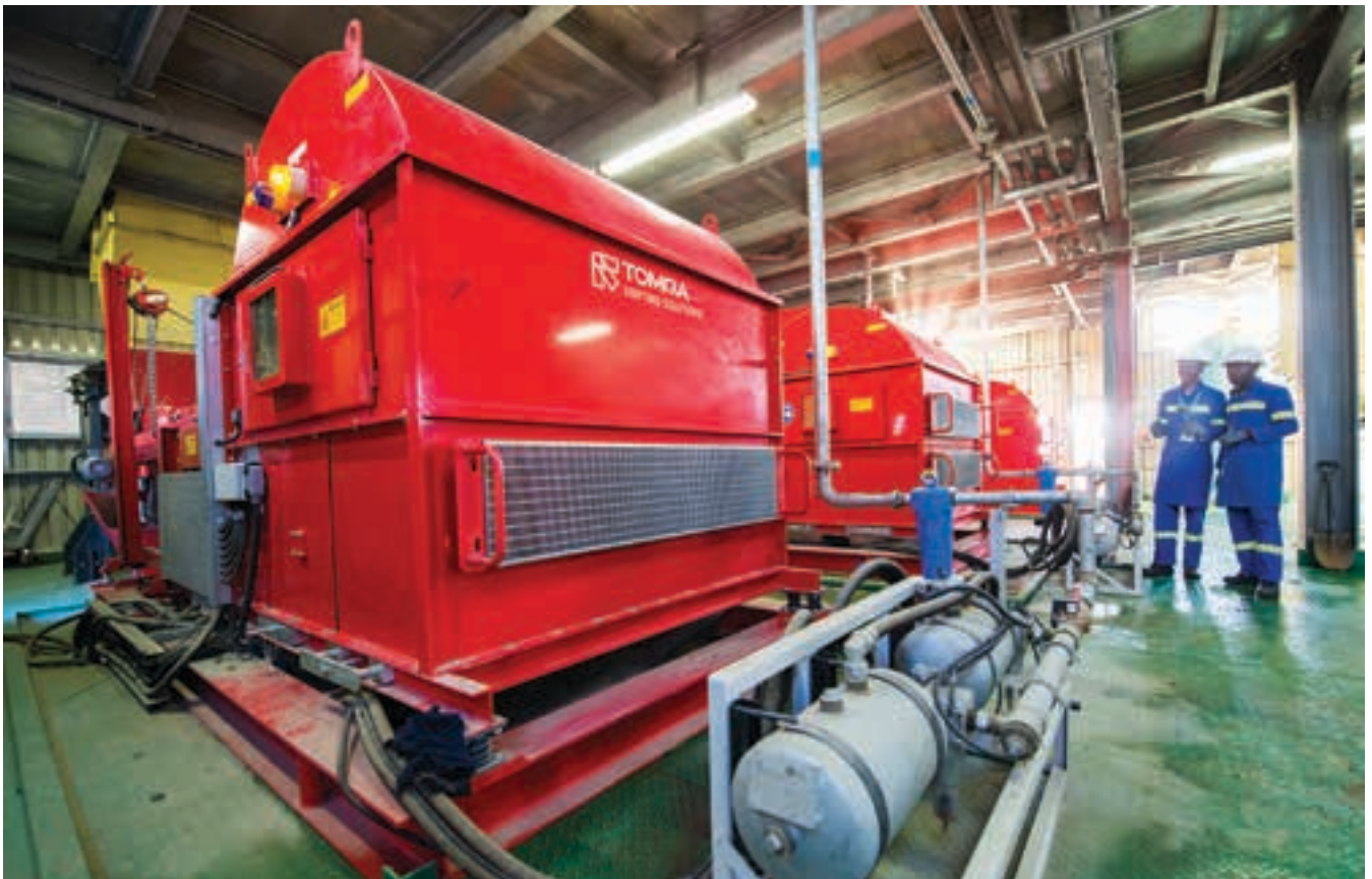
The TOMRA XRT machines installed at Karowe (photo: Lucara).
