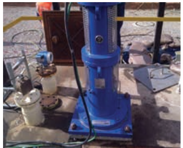
The Floway® VTP during installation at a customer's site.
