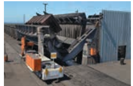
ELB has completed the refurbishment of the first tippler of the Transnet Tippler Refurbishment project at the Transnet Port Elizabeth Manganese Terminal.
