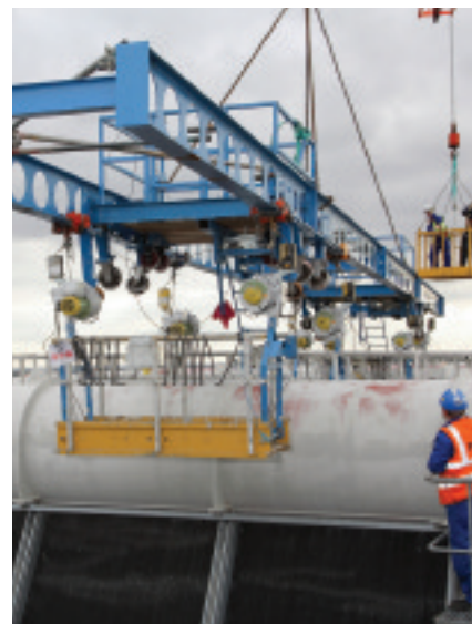
The access rigs being lifted into position on top of the ACC pipes
