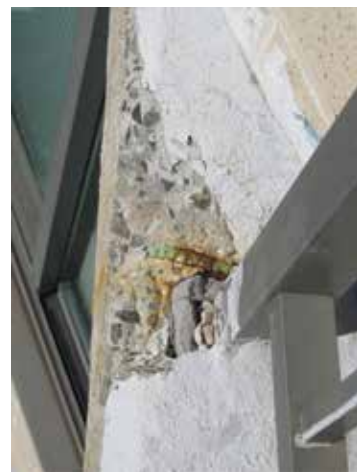
(above) Location of a "pitch pocket" where the handrail post is embedded in the concrete balcony. Moisture has entered the pocket causing rusting of the steel and cracking of the concrete.
