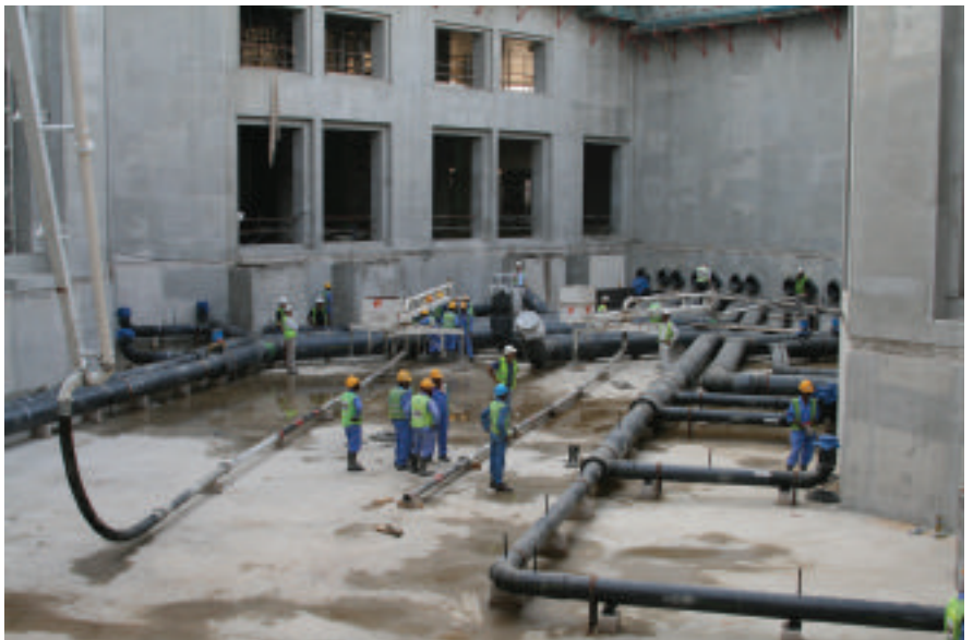
▲ Some of the larger diameter Uponor pipes during construction of the Atlantis Hotel aquarium
