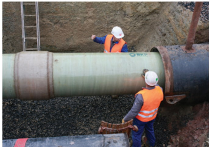
DN 1,200 casing tube (black), and BWP-coated steel pipe (green) with GRP spacer (brown)
