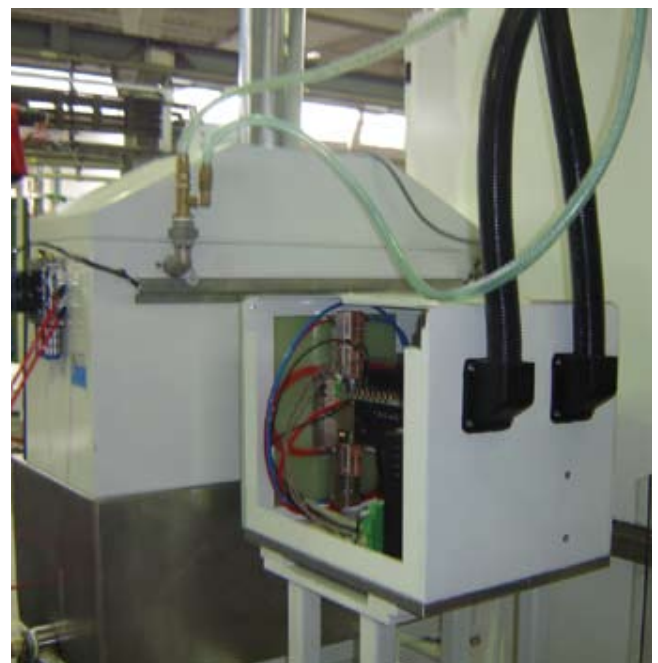
Figure 11: 30kW hardening generator
