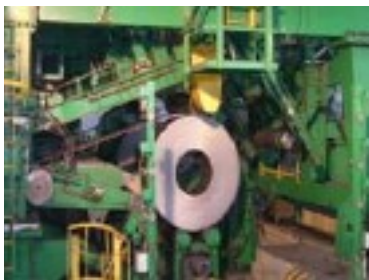
Automatic entry line
