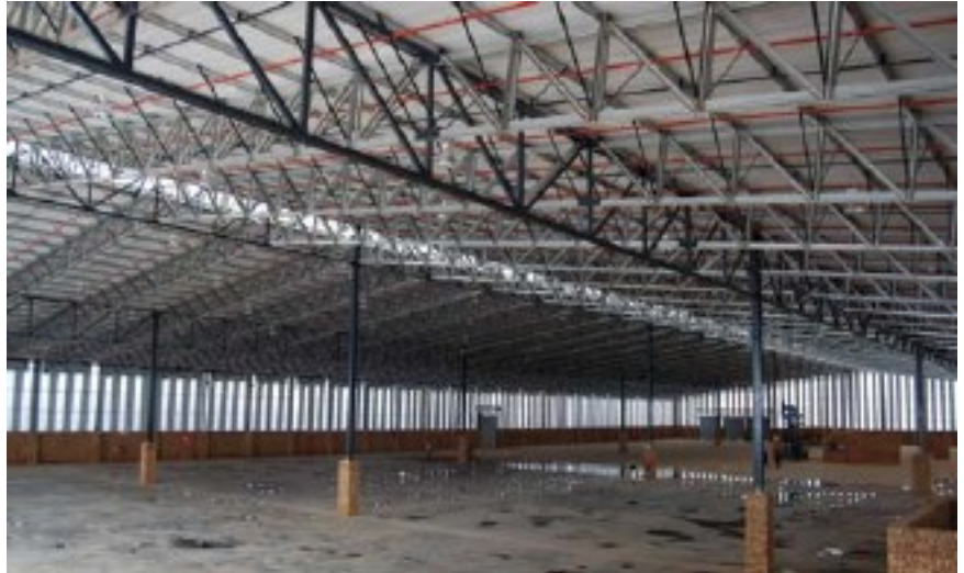
Using Robor Hybrid Structure, an 11,800m 2 factory was erected in just three months
