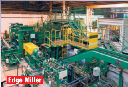
Coil handling equipment
