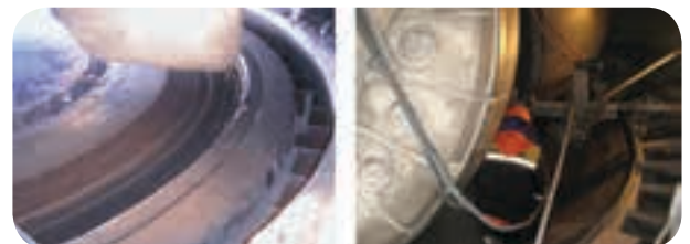
Figure 7: Left: Worn vertical mill table and roller and right: the flux-cored/metal cored welding equipment assembled for mill repair.
