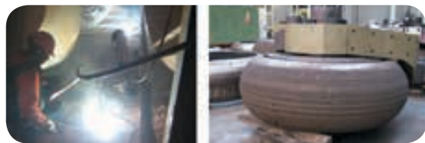
Figure 8: The repair of a vertical mill using SK 866-O (in situ) and (right) a mill roller hardfaced with SK A43-O flux-cored wire.
