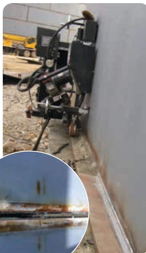
Above: A Lincoln LT7 tractor and Lincoln Flextec 650 power source is being used to complete the floor-to-shell outside circumferential weld using the submerged arc process. The same equipment is used to weld the tank base. Left: A completed AGW weld on a 20 mm bottom strake.
