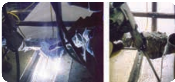
Figure 6: Repair welding of a kiln tyre using UTP 068 HH stick electrodes and peening of each bead following deposition.
